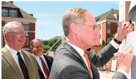
OSU President Burns Hargis signed the strobic fan as OSU A&M Regent Calvin Anthony looked on during the topping out ceremony for the Interdisciplinary Science Research Building.
